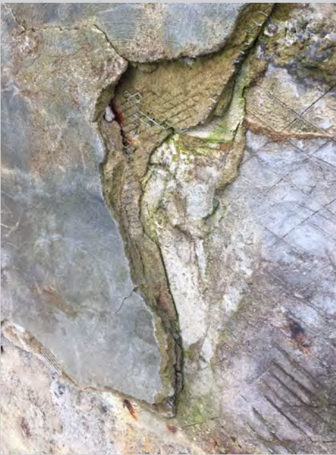
Damaged and hazardous wall prior to repair:
